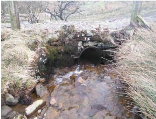
Photo 36. Existing culvert at water crossing 13 on Nant y Graig Lwyd tributary (SH 94700 05700)
