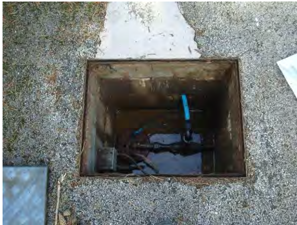
Photo 1. Private water supply for Dolwen (PWS 1)
