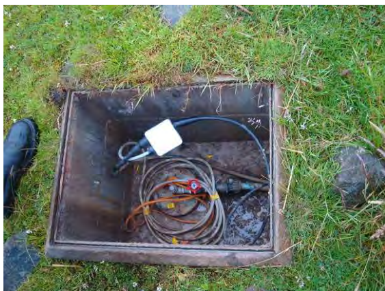
Photo 5. Borehole private water supply for Neinthirion (PWS 4a)
