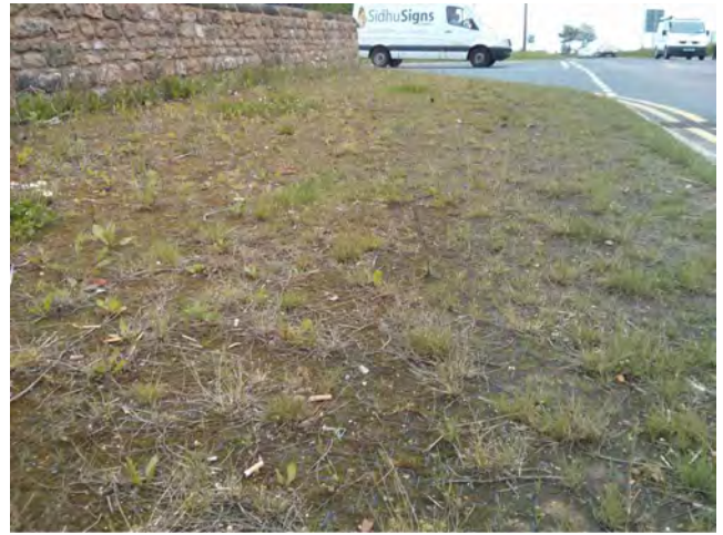
PHOTOGRAPH OF PERFO TERRA-GRID GRASS REINFORCEMENT AS PREVIOUSLY INSTALLED ON MARR WIND FARM, DONCASTER, PHOTO TAKEN 30.05.13
