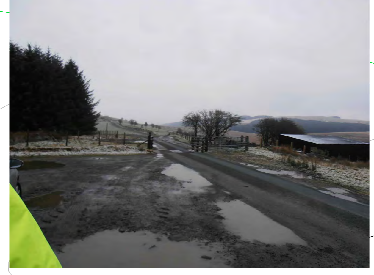
3.6 - EXISTING PASSING AREA CH 14250 EXISTING PAVED PASSING PLACE TO BE RETAINED. THE AREA IS NOT OF SUFFICIENT SIZE TO ACCOMMODATE HGVs.
