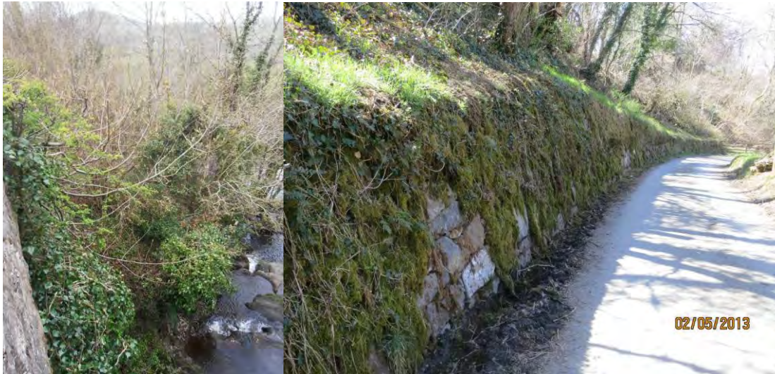
Photograph 6 - Existing foliage and embankment on the north western side of Gosen Bridge Photograph 7 - Existing stone retaining wall along the north western road down to the river
